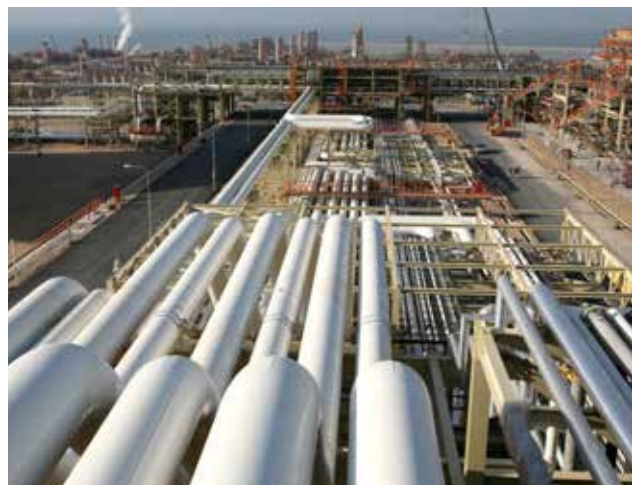
Transocean paints protect onshore- and offshore facilities in the world largest gas reserves: the South-Pars Gas Fields.
